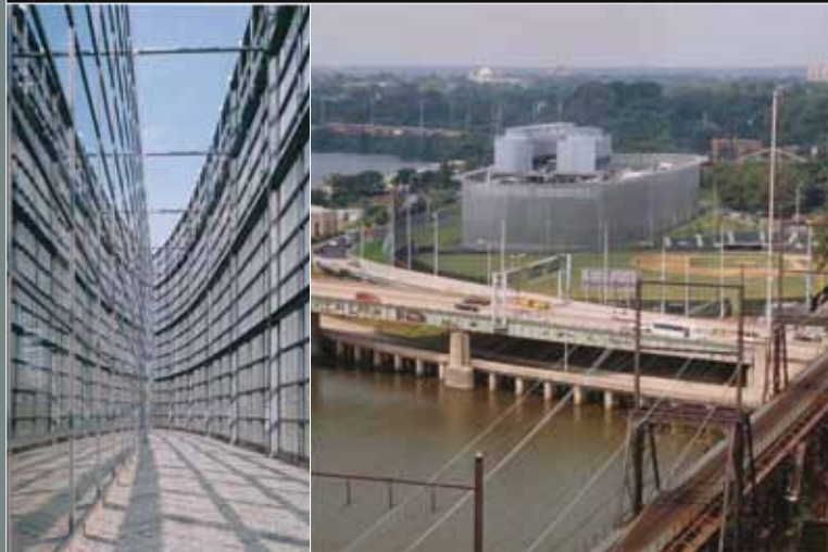
University of Pennsylvania, Gateway Chiller Plant
